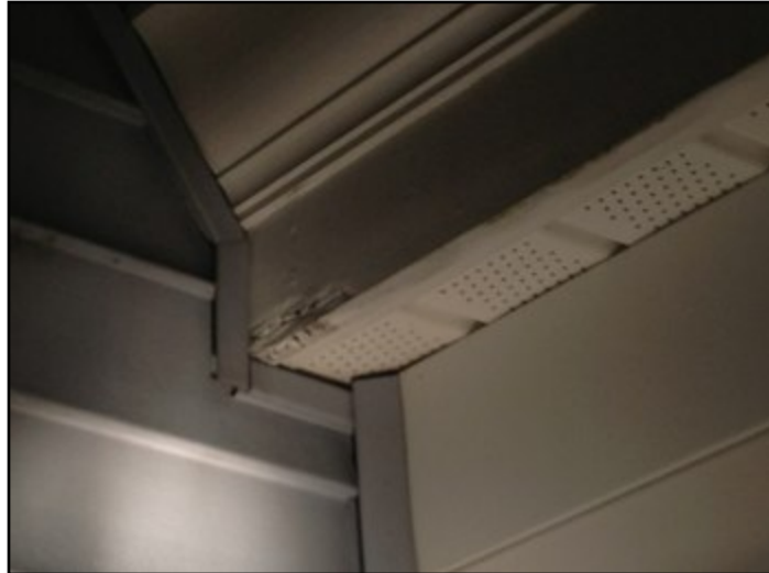
1. No gutters or downspouts
